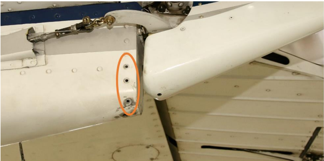
Figure 3-8, Aft Bulkhead LH Rivets, Removed
